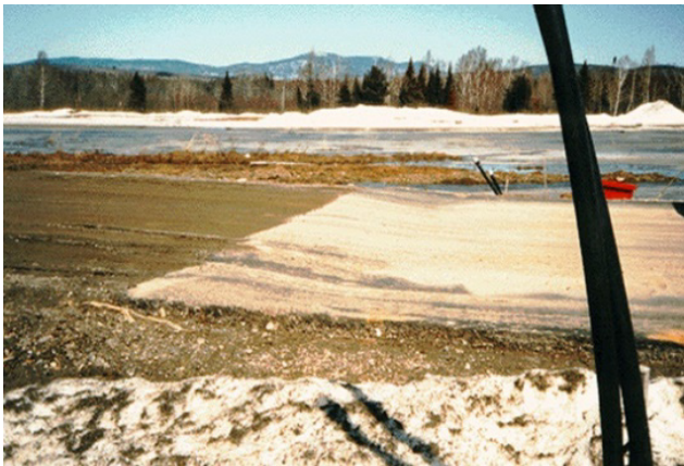
a. Example of heave as a result of no insulation.
